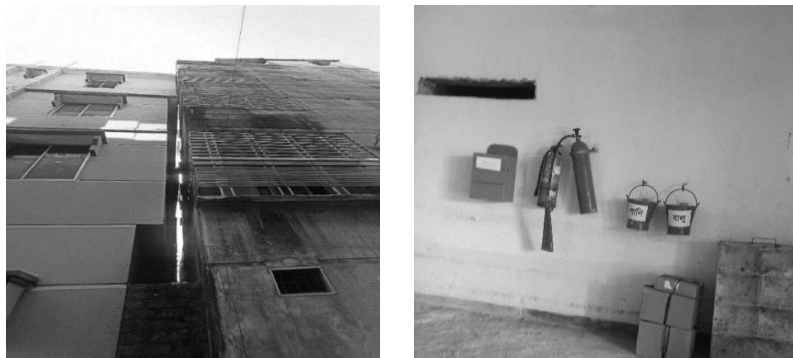
Figure 3. Building to building distance and fire extinguisher
