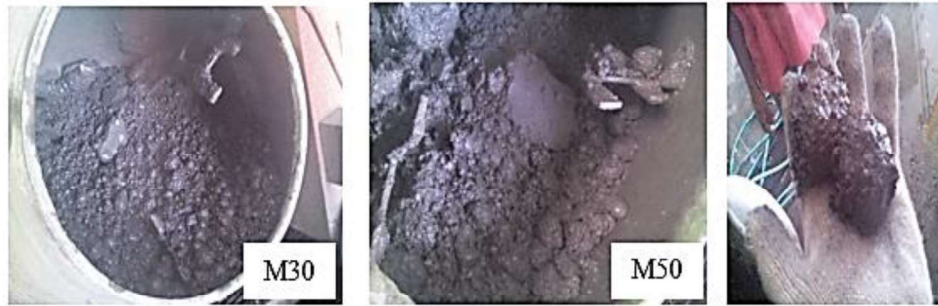
Figure 4. Mixes M30 and M50 in a concrete mixer machine at lower superplasticizer content.
