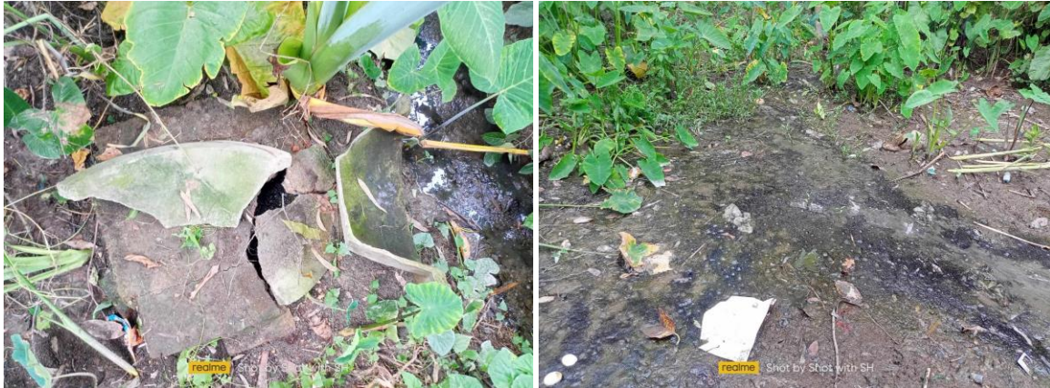
Figure 9. Septic tank effluents discharge nearby depression
