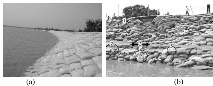
Figure 7. (a) Geo Bag Dumping for river training (b) Failure in geobag revetment (1 = pullout; 2 = slump; 3 = dislodgement of top bag; 4 = slide; 5 = physically damaged) (Akter, A., et al., 2009)
