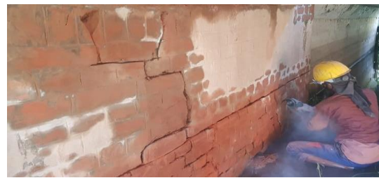
b) Horizontal and vertical cracks in Abutment (221 up)
