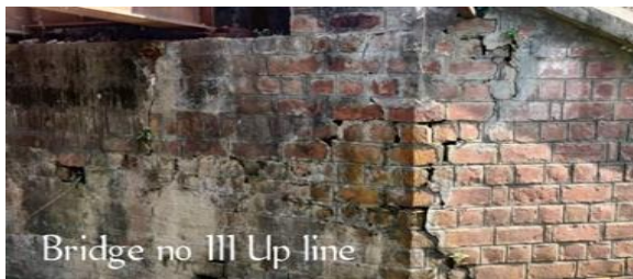
a) Cracks in Bed block, abutment, and wing wall (111up)
