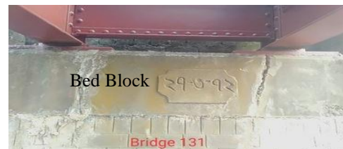
d) Cracks in Bed block (Bridge No. 131 dn)
